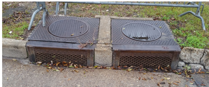
Figure 3-9 Catch Basin Screen Example
